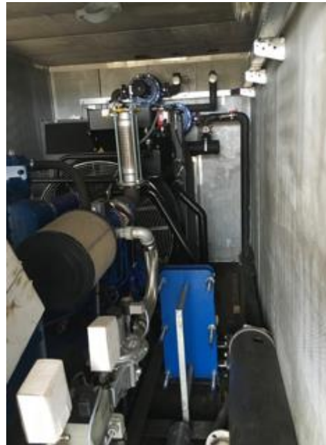
CHP installed and operational 100KW
