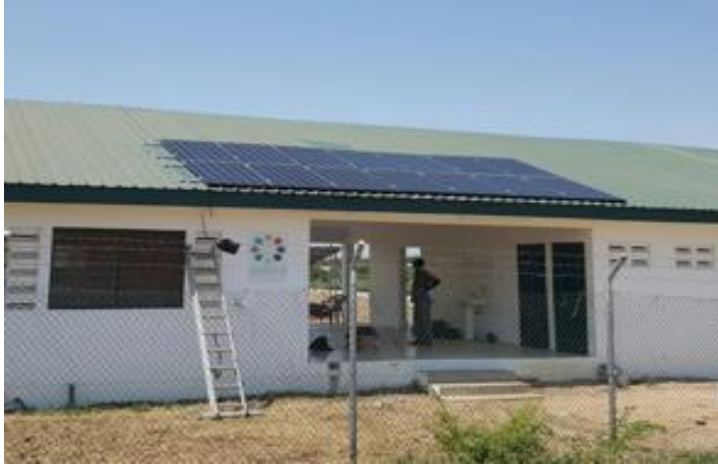
New solar panels at office 3.5 kWh (peak)
