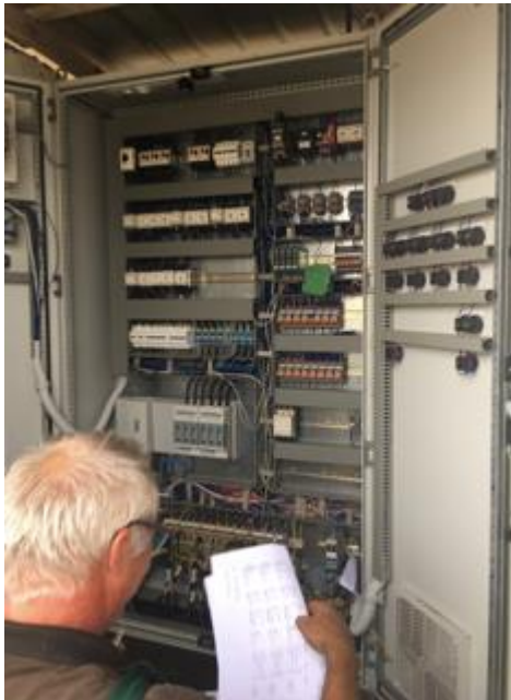
Switch board checks by supplier
