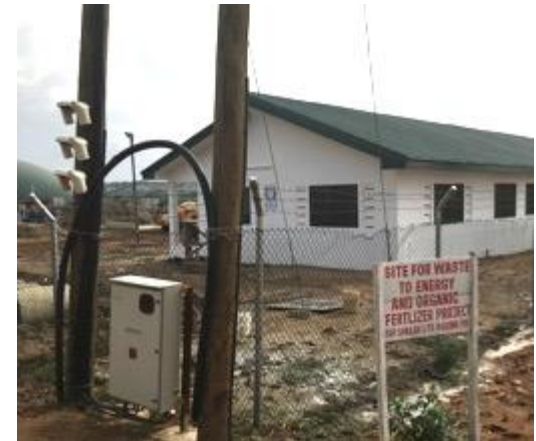
Connection to grid and main meter
