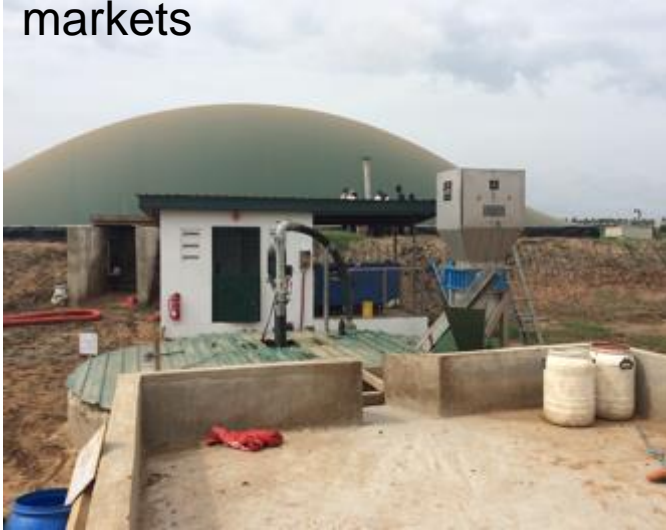
Mixing pit (faecal and organic waste) + macerator + digester
